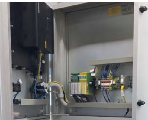
Assembly and wiring
